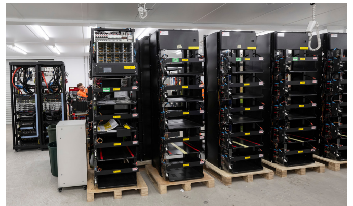
Enatel customised solutions for Indoor Hybrid and SP36 cabinets ready for final testing at Battery Energy Configuration Centre in Sydney, prior to shipping to customer.
