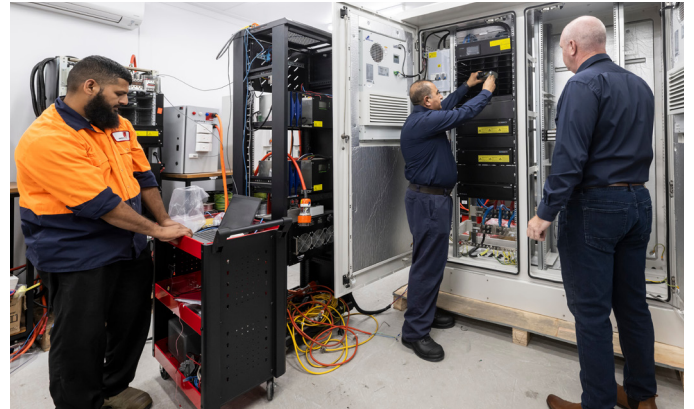
Enatel Hybrid System installed in Battery Energy Dual Bay outdoor cabinet in Battery Energy Configuration Centre, Sydney.
